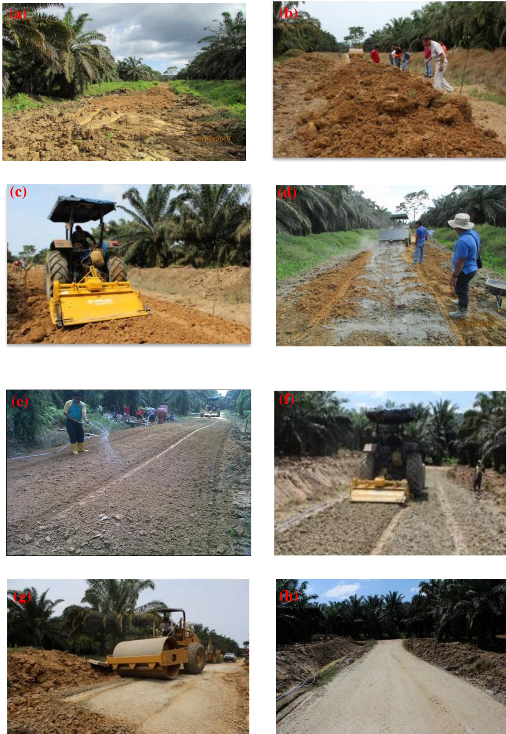
Figure 5. (a) Skimming the soft layer of road surface; (b) Importing quality soil from nearby area; (c) Rotovating the surface soil; (d) Distributing additive premix on road surface; (e) Watering the prepared surface; (f) Rotovating the prepared surface; (g) Compacting the prepared surface; (h) Completed treated road.
